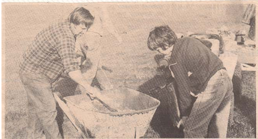
Del Fisher (left) and Mike Newton mix cement for fence construction at new Little League fields. Opening ceremonies at the fields are scheduled for April 25.
